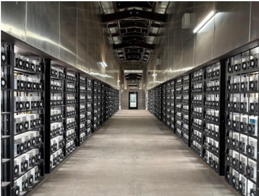
Mining rigs energized and hashing at Black Pearl
