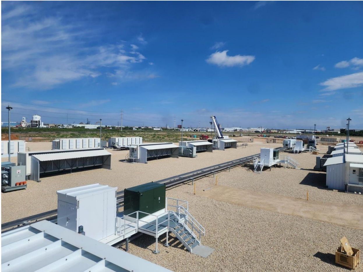
Odessa Data Center Area A – Awaiting Arrival of Canaan Rigs
