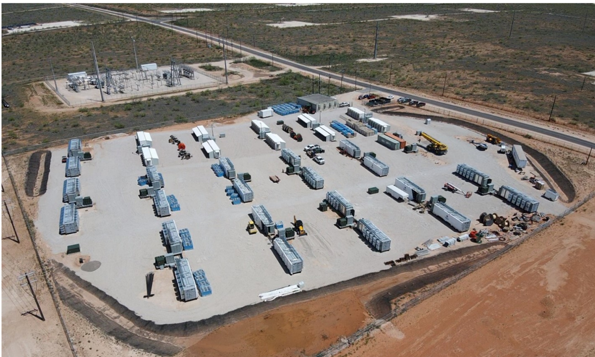
Completed infrastructure at Bear with 30 MW expansion on track for Q2 2024 energization
