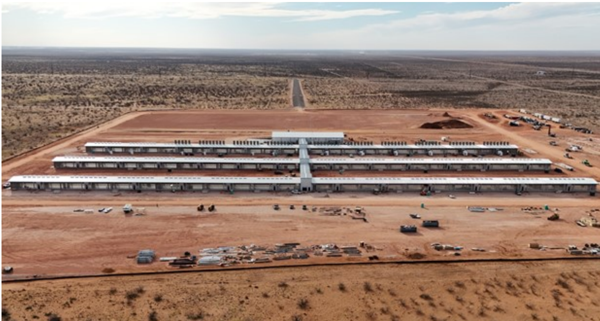
Construction at Black Pearl site. Each of miner wings 1-3 is ~1,000 feet long and will hold approximately 13,440 mining rigs.
