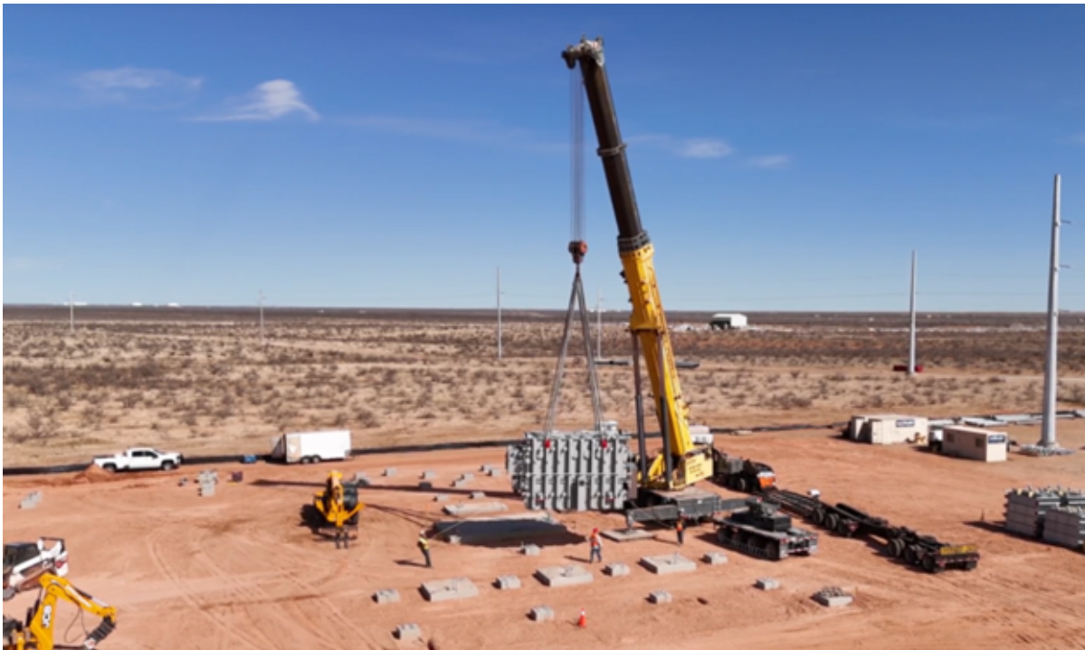
Recent arrival of the first substation transformer at our Black Pearl site.
